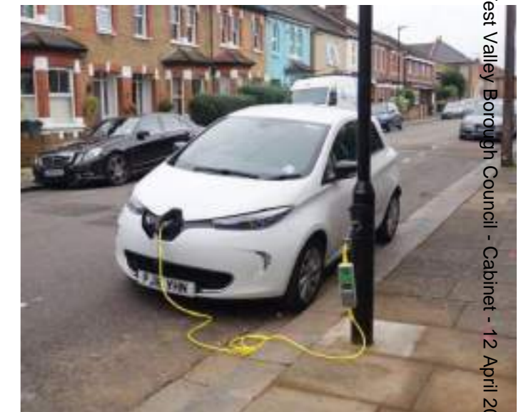
Residential lamp column charging / London
