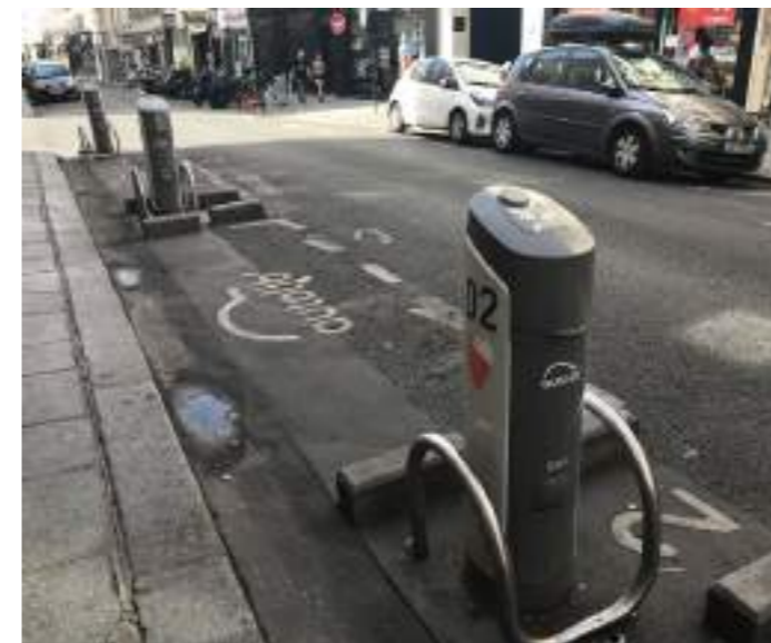
Efficient & unobtrusive charging banks / Paris
