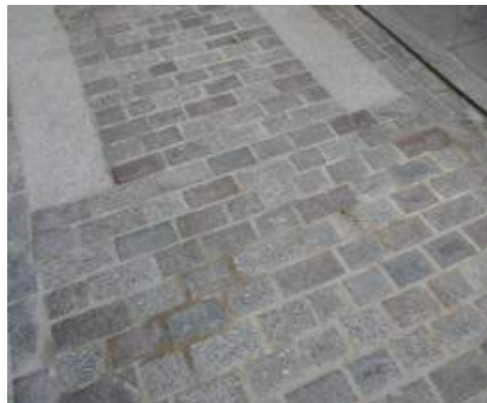
New laid kerbs / with two courses of setts laid longitudinally to form channels within the carriageway draining to traditional gully points in White Hart Yard, London
