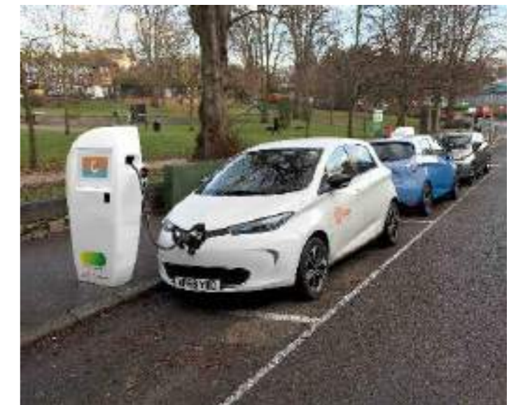
Unacceptable placement of chargers / Devon
