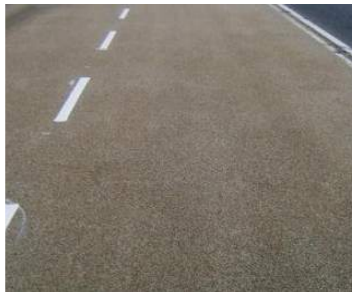
Hi-friction slip resistant resin bonded aggregate / applied to wearing course provides a lighter surface and helps prevent traffic accidents.
