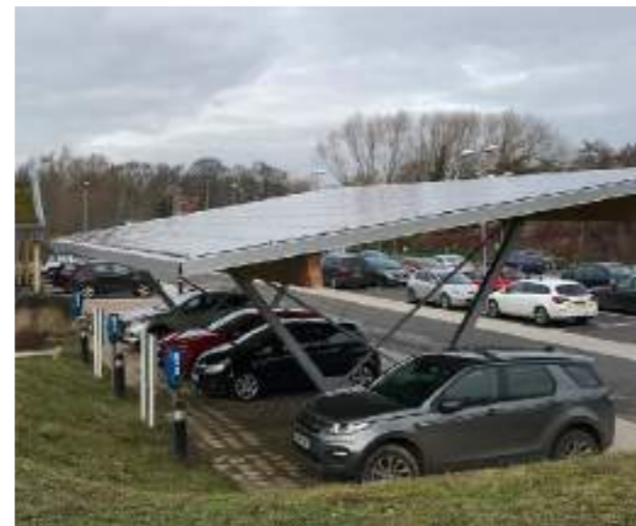
Charging within car parks, using solar
